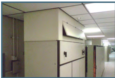
Filter Access Doors
