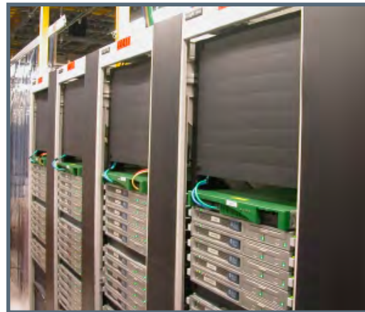
Fill Gaps Between Racks
