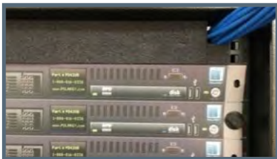
Blanking inside racks
