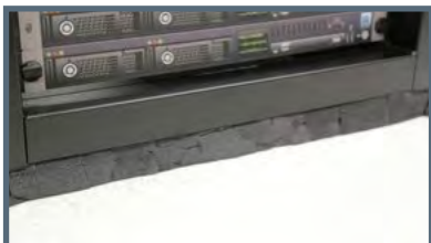
Above, below and between racks
