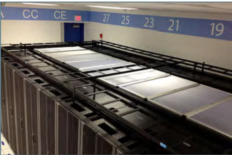
Drop Away Panel Roof on APC Cabinets
