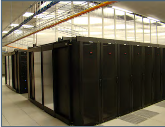
Hot Aisle Containment
