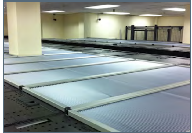
Cold Aisle Containment
