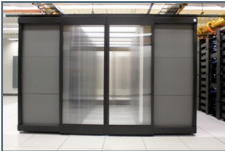
Cold Aisle Containment
